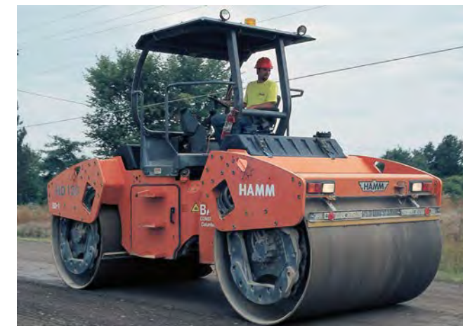
Hamm HD 120 roller provides finish compaction for local traffic on reclaimed road base
